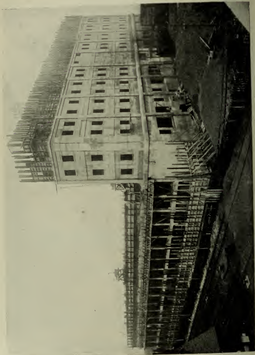
MOVING FORMS AT THE KING GEORGE DOCK, HULL. (See p. 459.) [Side view of bins, showing the moving forms. One concreting wagon is seen at work, and the jacking crew may be discerned in the background.]
